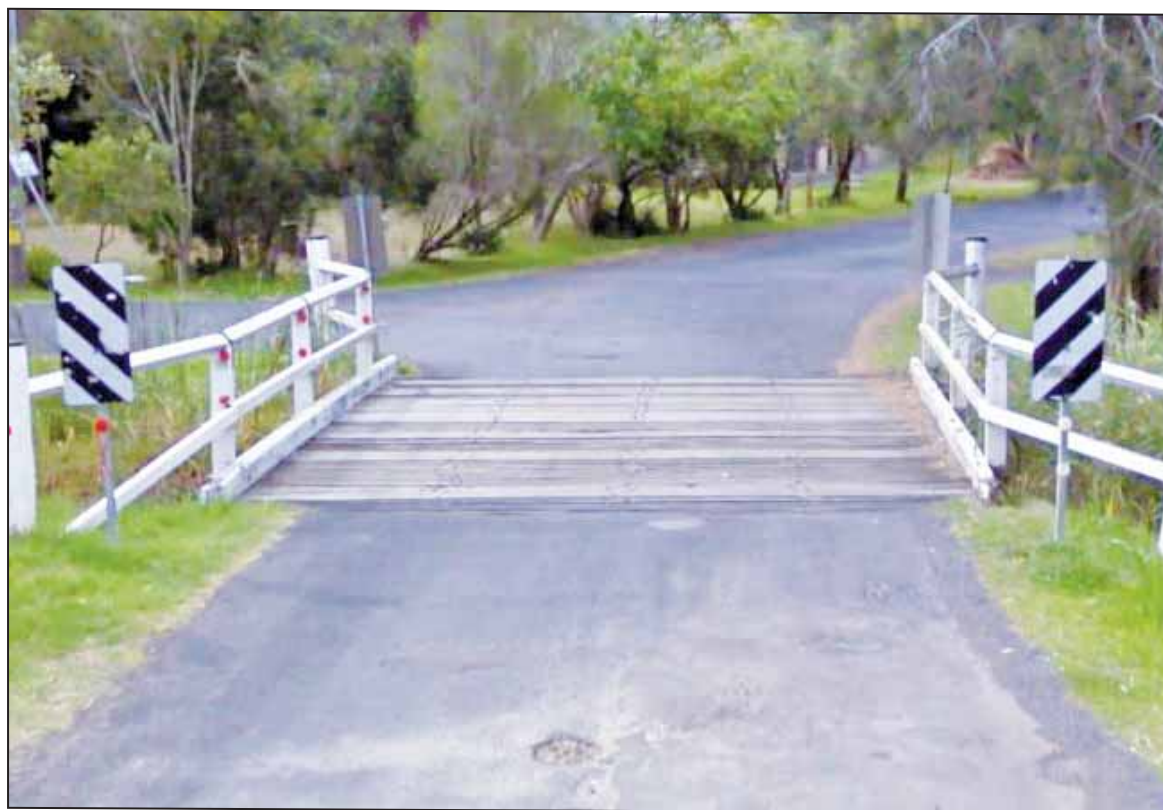
The bridge at Noble Rd under which the sewage spill was first noticed
