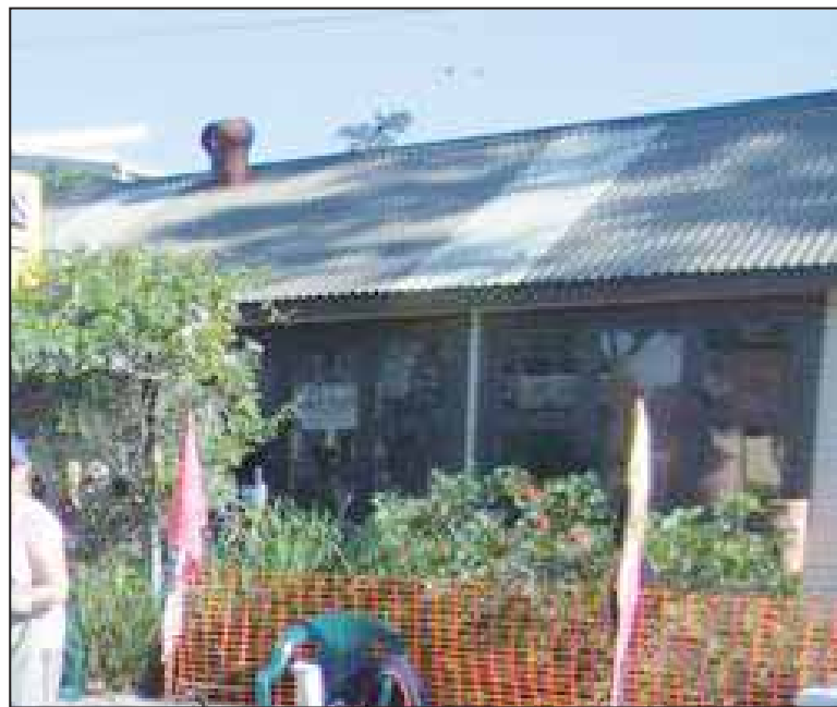
The old roof of the Ettalong Beach Arts and Craft Centre's pottery building
