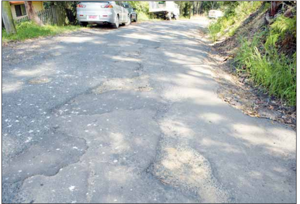
Potholes on Phegans Bay Rd
