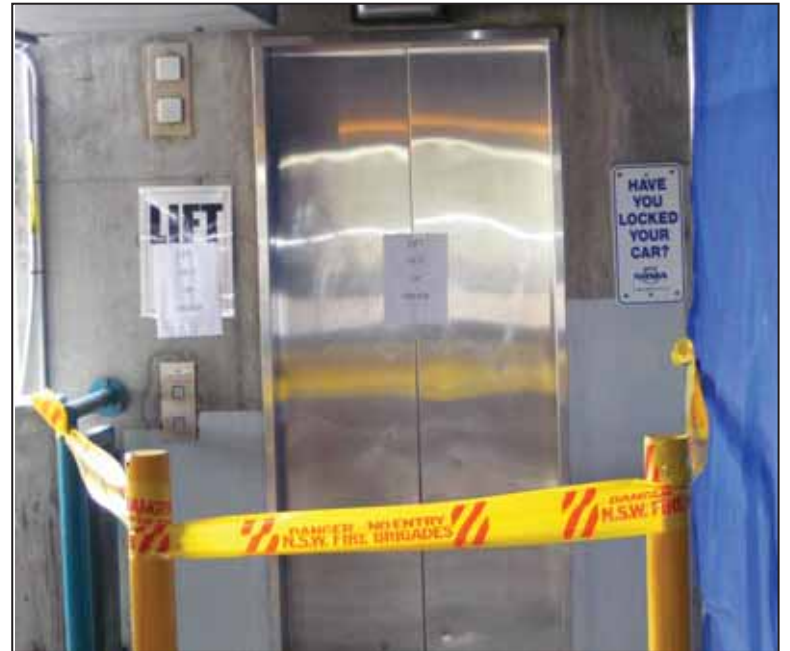
The damaged lift at Woy Woy commuter car park
