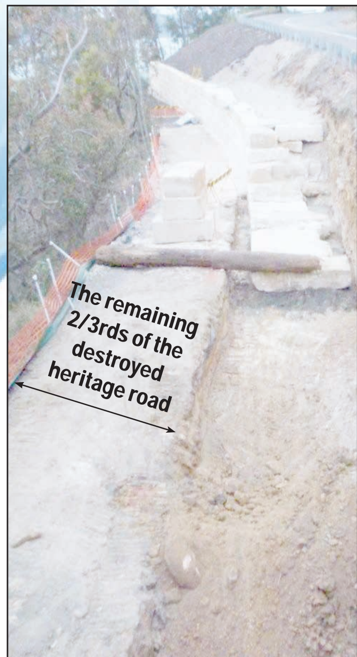
This photo leaves no doubt that Gosford Council permitted the trashing of a heritage road and the building of a much larger than needed retaining wall to simply silence community calls for the return of a road around the point from Umina to Pearl Beach.
