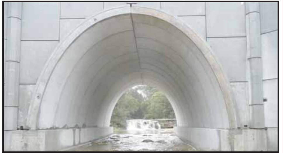
After: Piles Creek overkill, memorial to 'human error'
