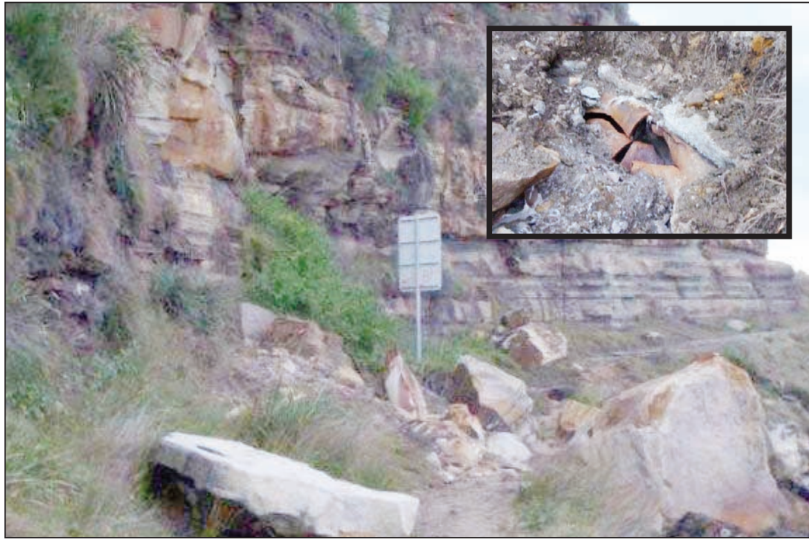
Rockfall breaks rising sewer main (Photo: Ed James)
