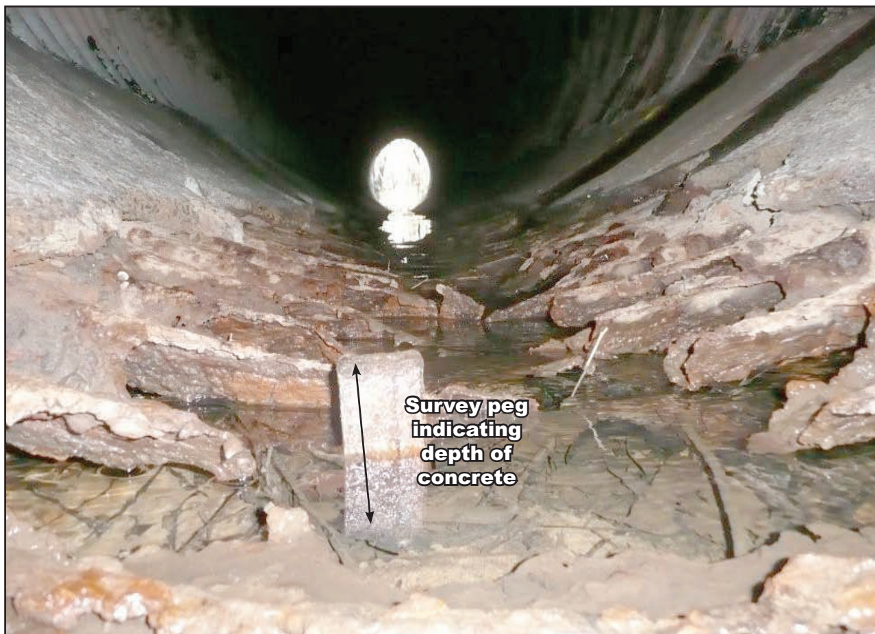
This photograph shows evidence the concrete was used during construction and again as maintenance later in two pipes located in the upper reaches of Mooney Mooney Creek beneath Peats Ridge Road
