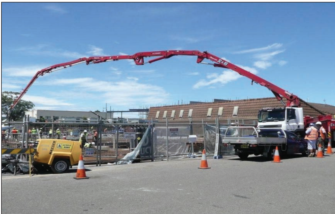
Construction workers onsite at the new Woolworths supermarket development in Umina CBD
