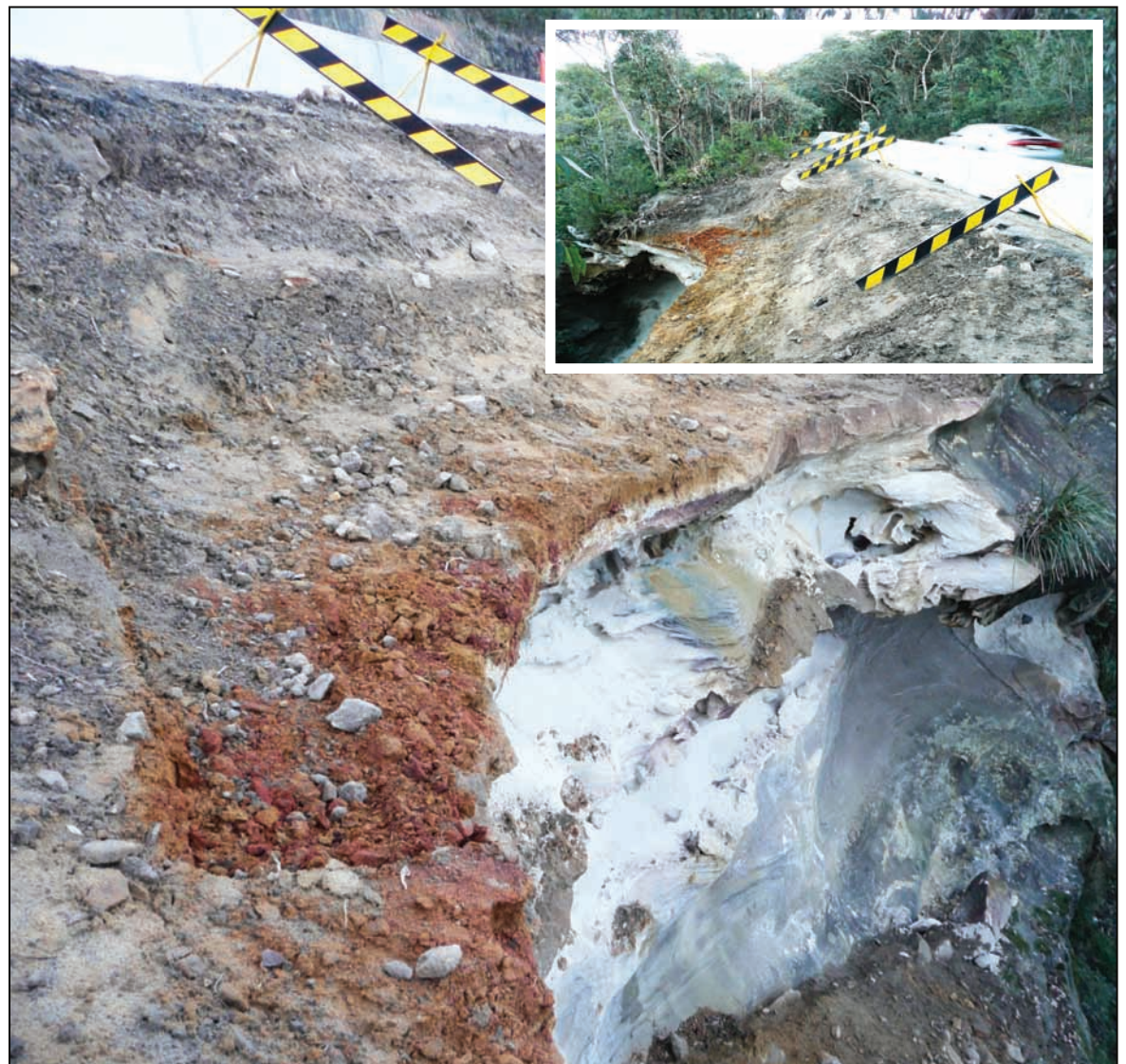
The site along Woy Woy Bay Rd where a section of rockface collapsed onto bushland and roadway above Phegan's Bay Rd (photos courtesy Mr Edward James)
