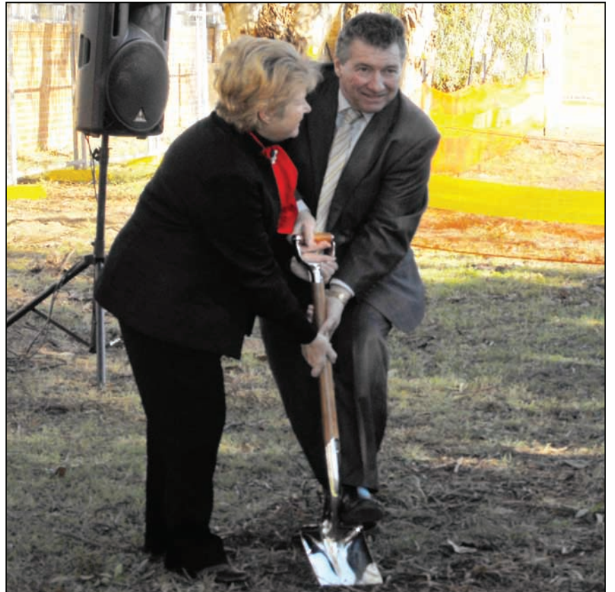
Member for Gosford Marie Andrews and Member for the Central Coast John Della Bosca turn the first sod for construction of the new trade school at Woy Woy Campus
