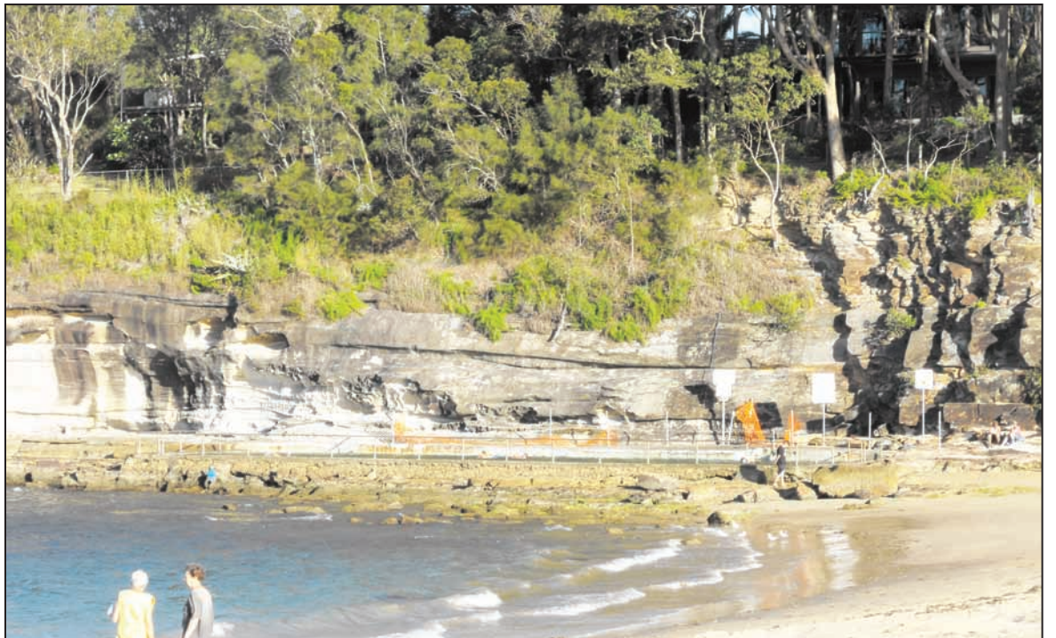
The cliff face near the Pearl Beach Rock Pool will undergo $140,000 worth of stabilisation works to make the area safer for locals and visitors to the area
