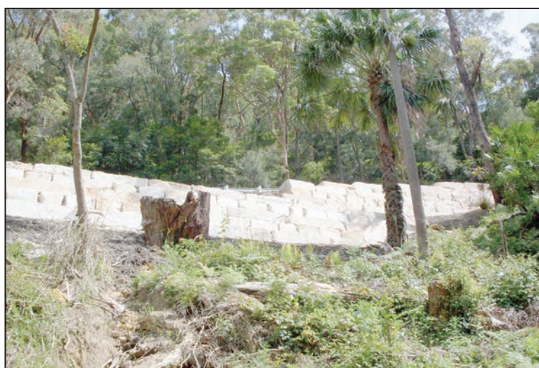
Slip repair work carried out by Gosford Council following the partial road collapse on Woy Woy Rd in April this year
