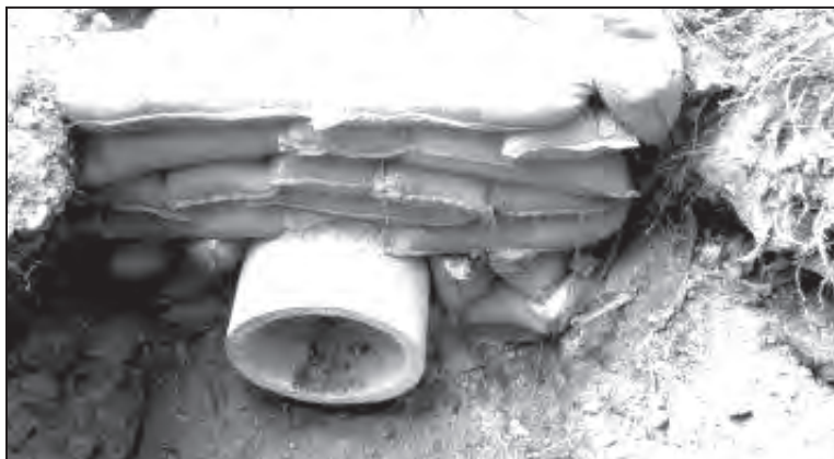
Council works being undertaken at Pearl Beach Dr (photo courtesy of Edward James)
