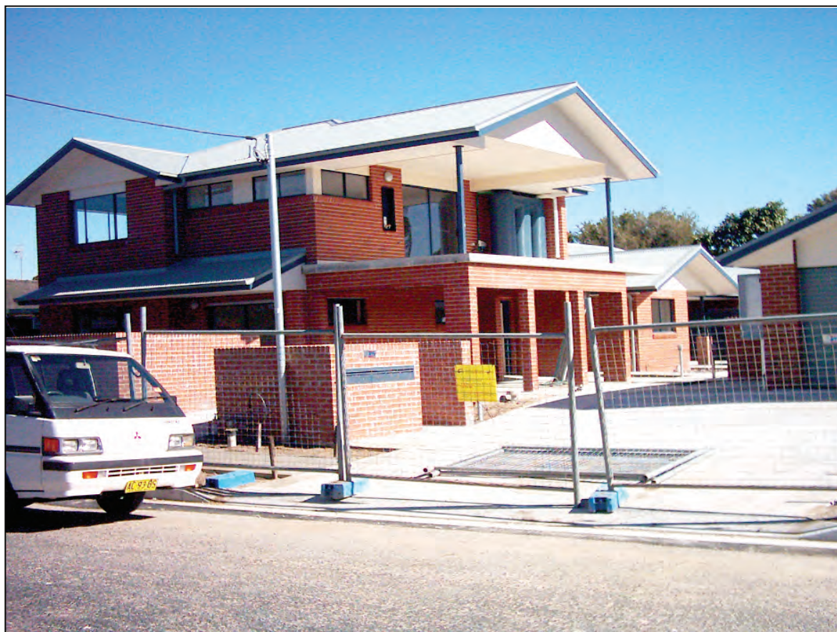
The State Government's affordable units being constructed in Daffodil Dr, Woy Woy
