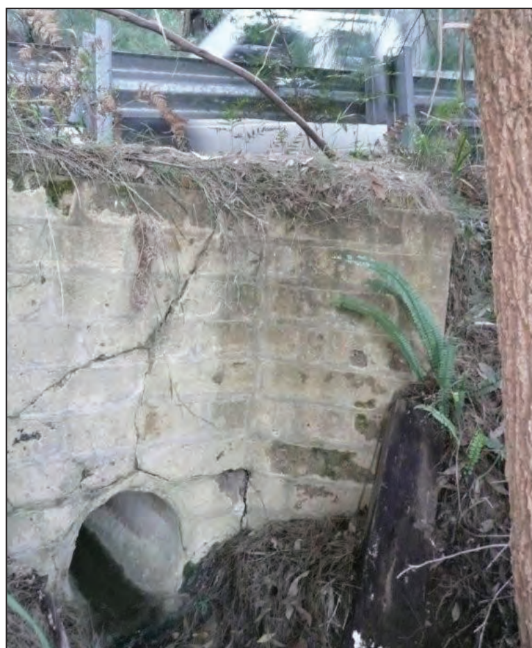
A cracked culvert under Pearl Beach Dr, Pearl Beach
