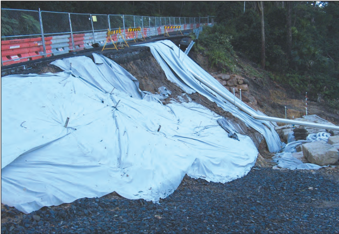
Work takes place on the collapsed section of Woy Woy Rd Bulls Hill
