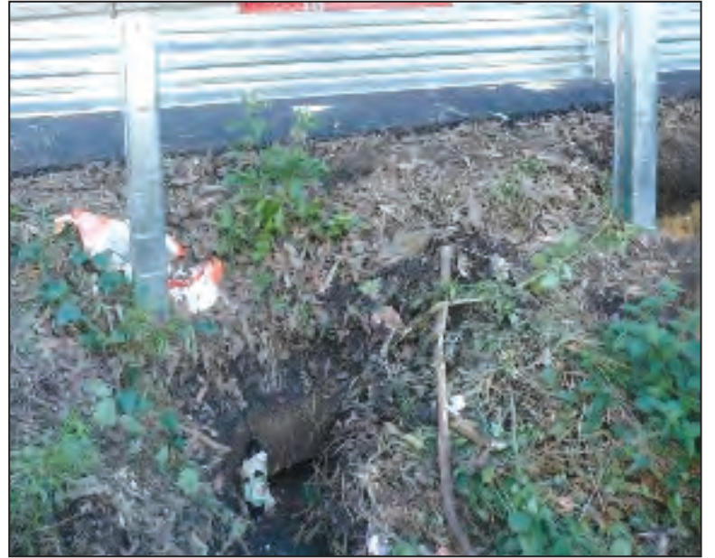
The blocked drain after the collapse on Woy Woy Rd;
