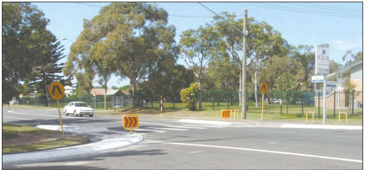
Upgrade work has begun on the pedestrian crossing at Umina Public School
