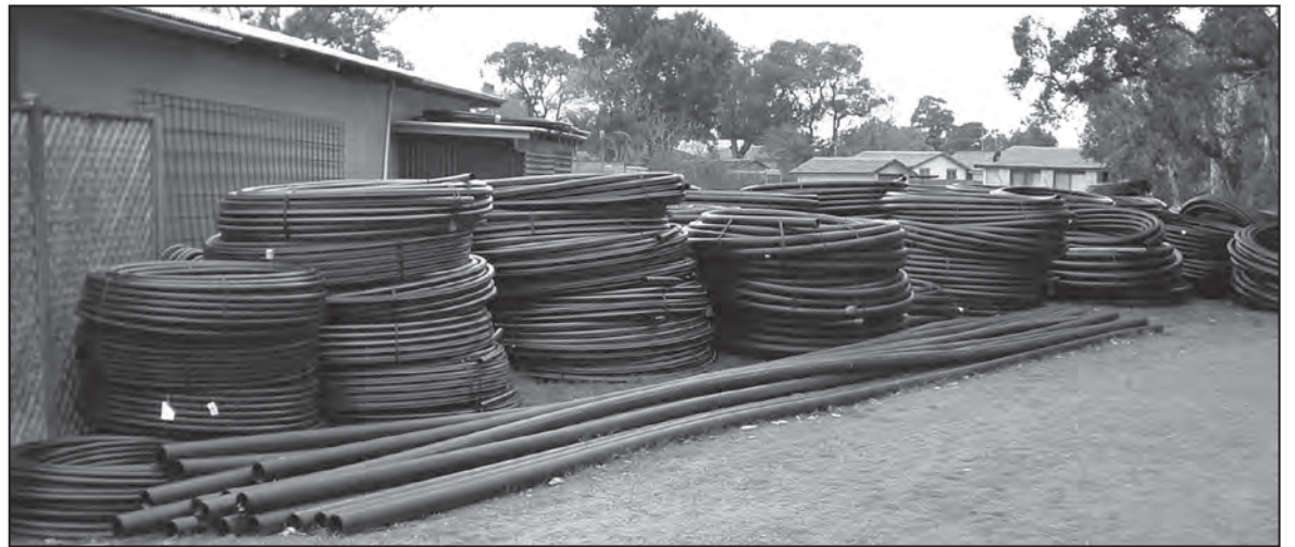
Irrigation piping before it was laid at Everglades Golf Course in September 2004
