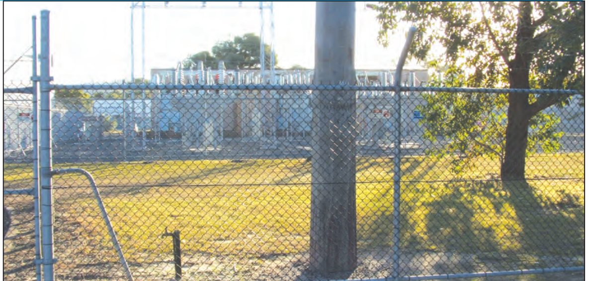
The Woy Woy Substation on Ocean Beach Rd, Woy Woy
