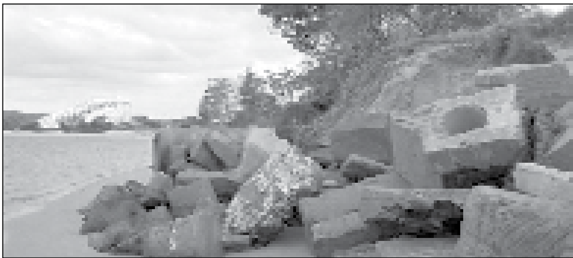
Erosion on the Ettalong foreshore during March this year
