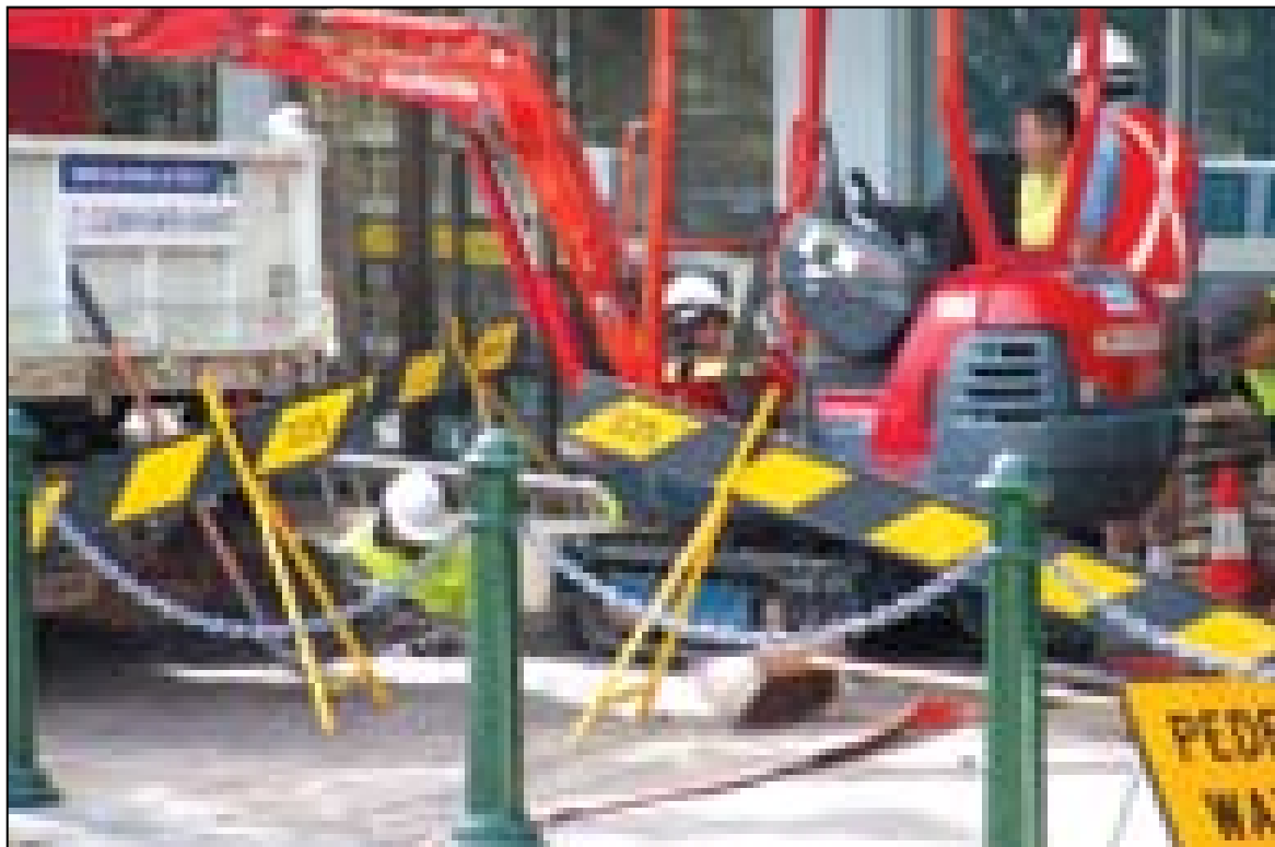
Council officers working on the broken water main outside Simplicity Funerals on Blackwall Rd, Woy Woy
