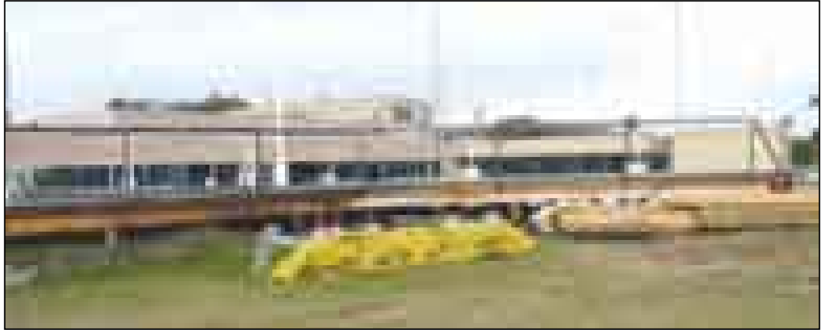
The dek outside the Woy Woy Bowling Club, where work has recently been halted
