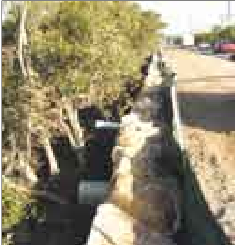
The new bike path being built on Brisbane Water Dr, Woy Woy
