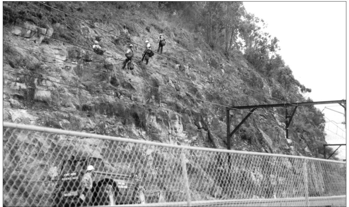
Railway workers at Koolewong clear the cliff face of debris to prevent falling rocks from striking trains
