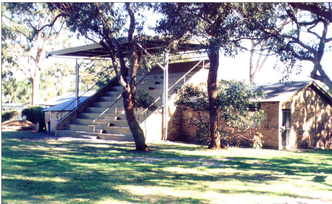
The condemned grandstand at Ettalong Oval
