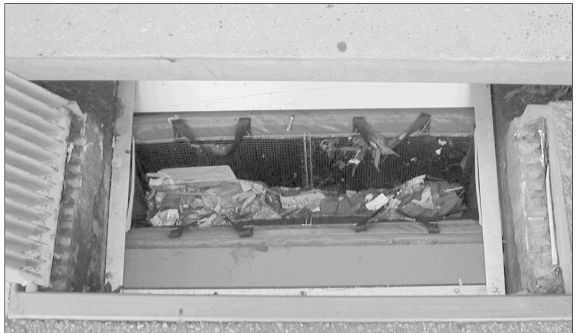
A drainage litter trap full of rubbish soon after installation
