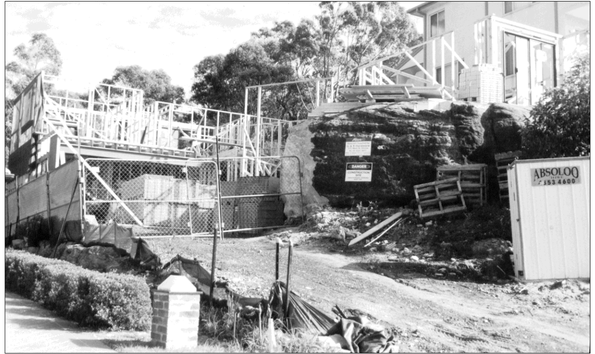
The house under construction at 36 The Citadel, Umina will not comply with the council DCP
