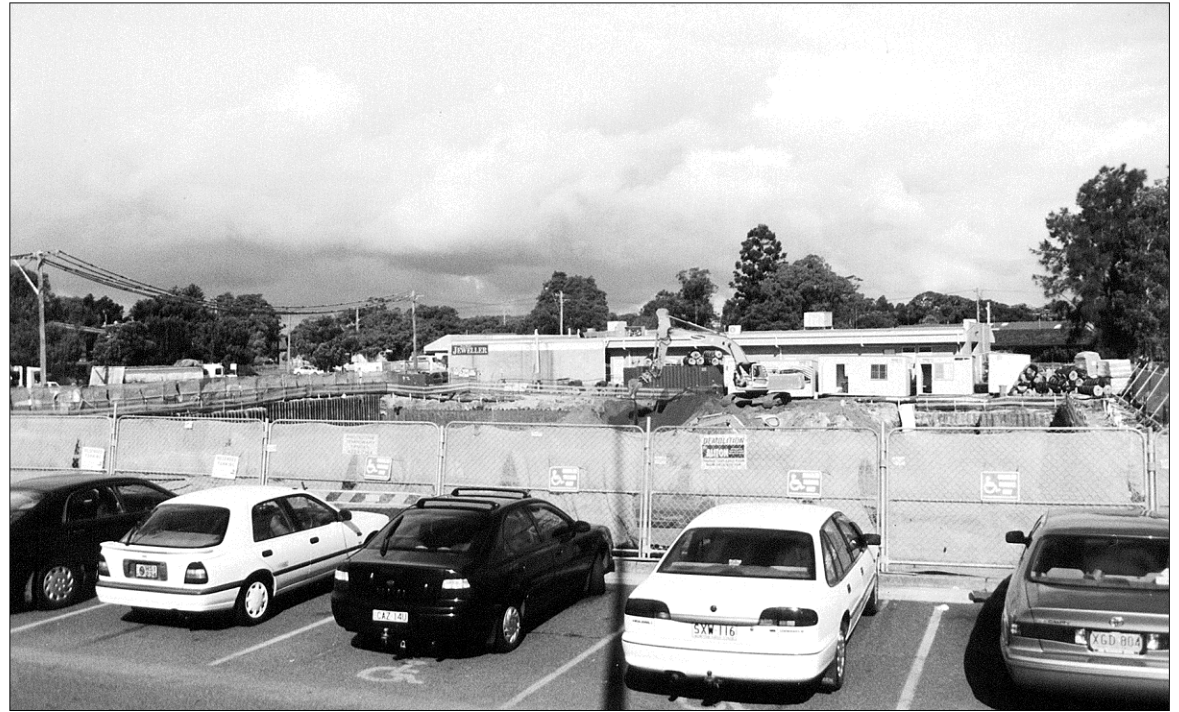
Work is underway on the new retail and commercial building on George St next to Deepwater Plaza
